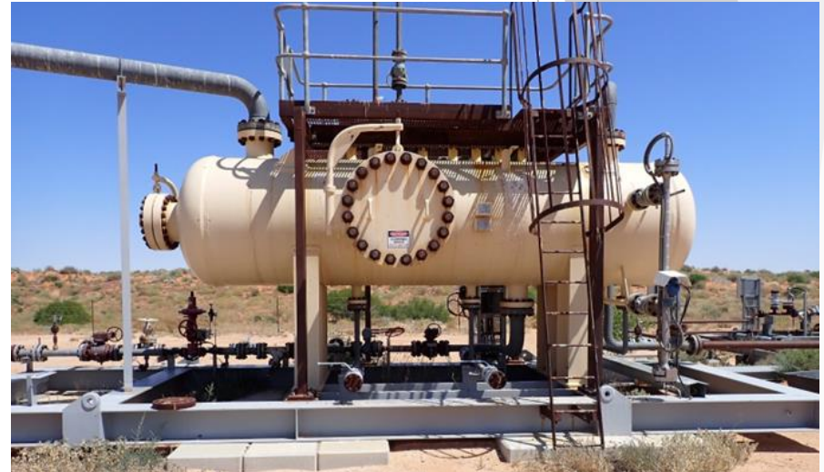
Figure 3: Gas/liquids separator in place at Vanessa facility
